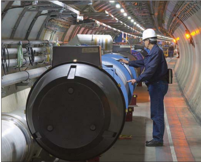
As far as the eye can see – magnets are now filling the LHC tunnel.
